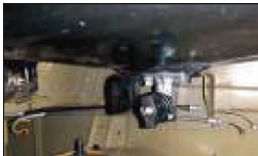
A. Fuel Tank
